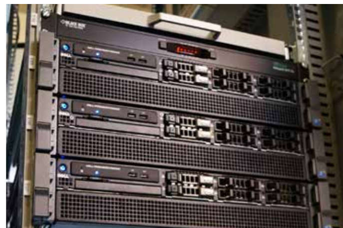
Inside the server cabinet for Optimal PAT solution for pharmaceutical production.
